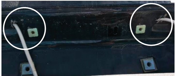
Factory-installed lights removed, with holes left uncapped. New holes added to accommodate after-market wiring.
